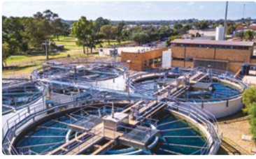
Water treatment plant, Mildura
